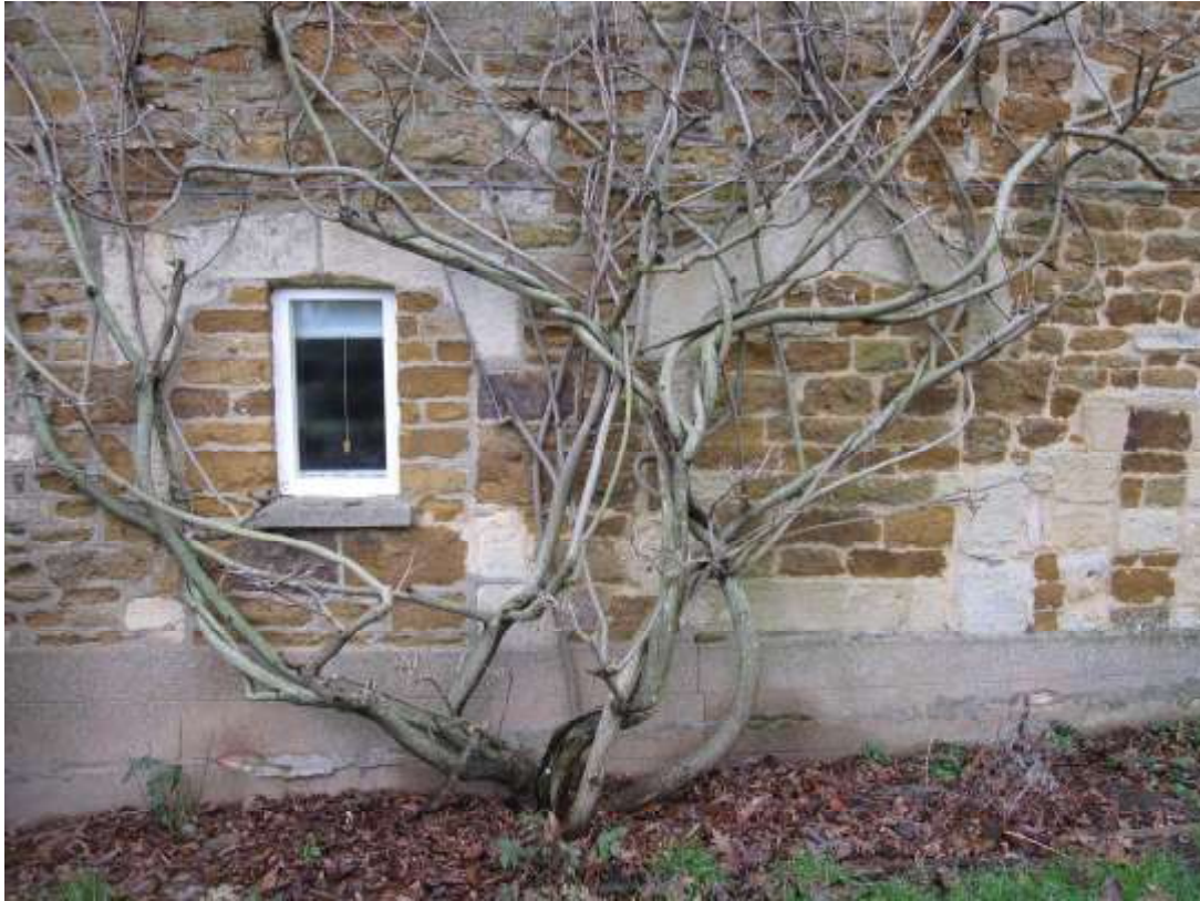
West gable with blocked medieval service doorways and slit opening to south
