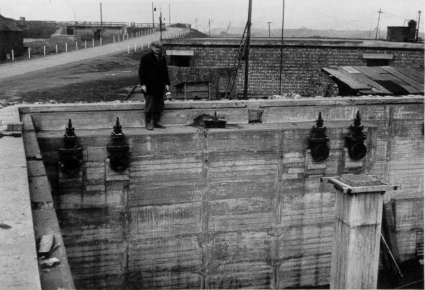
9"Sluice Valves, before ball valves are added. Mr. Simpson, Clerk of Works.
