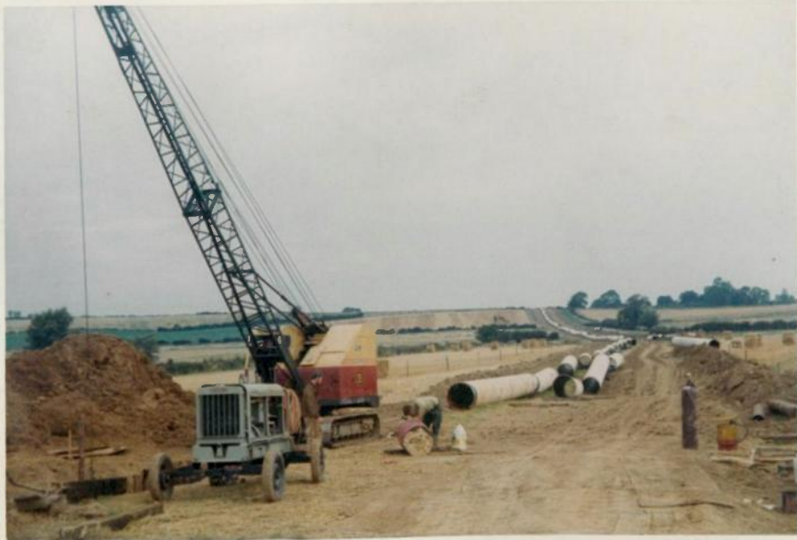
36" dia. North Sea Gas line taken from the Eye Brook approach road.
