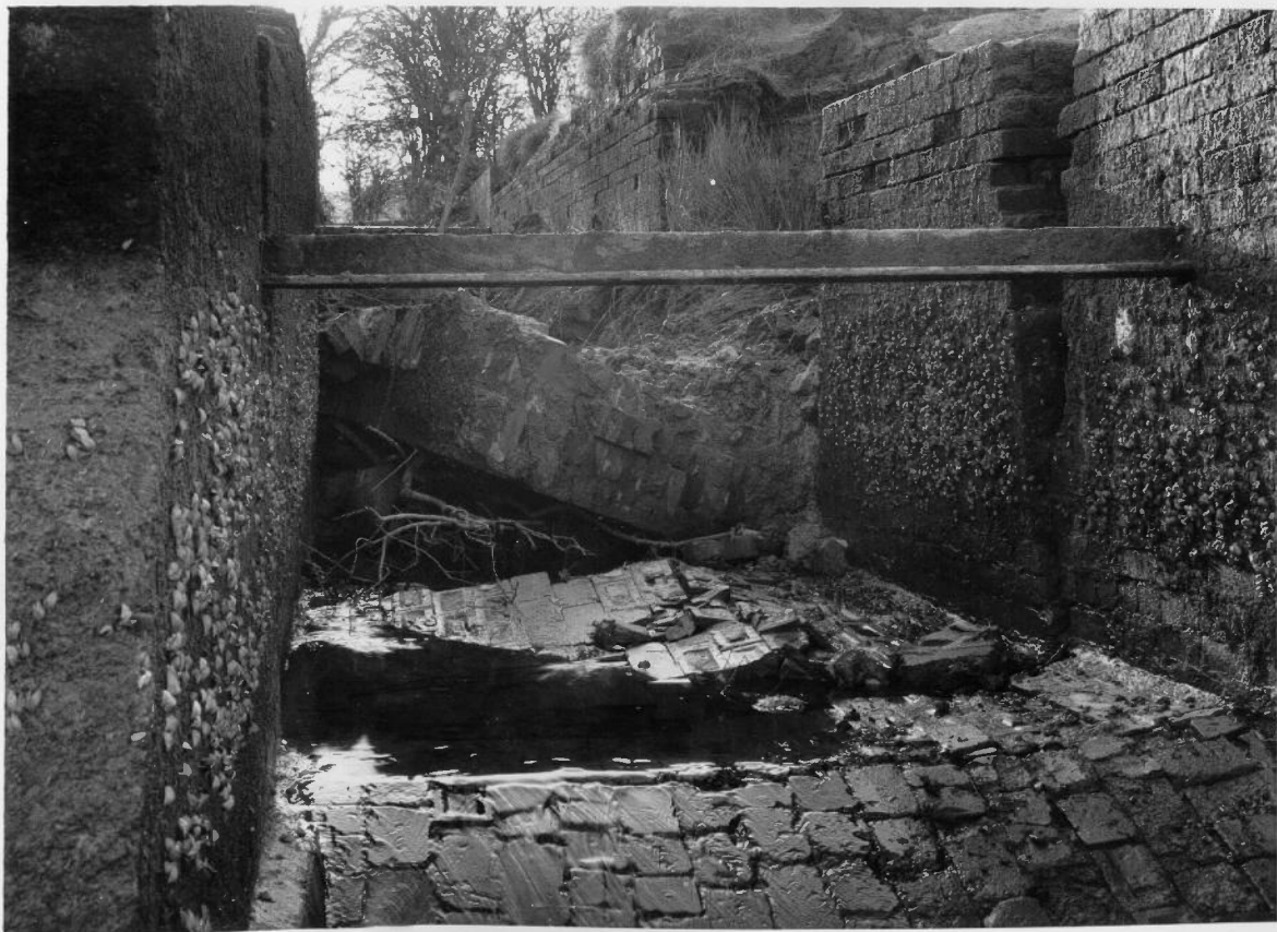
Broken Clayhole culvert. December 1961.
