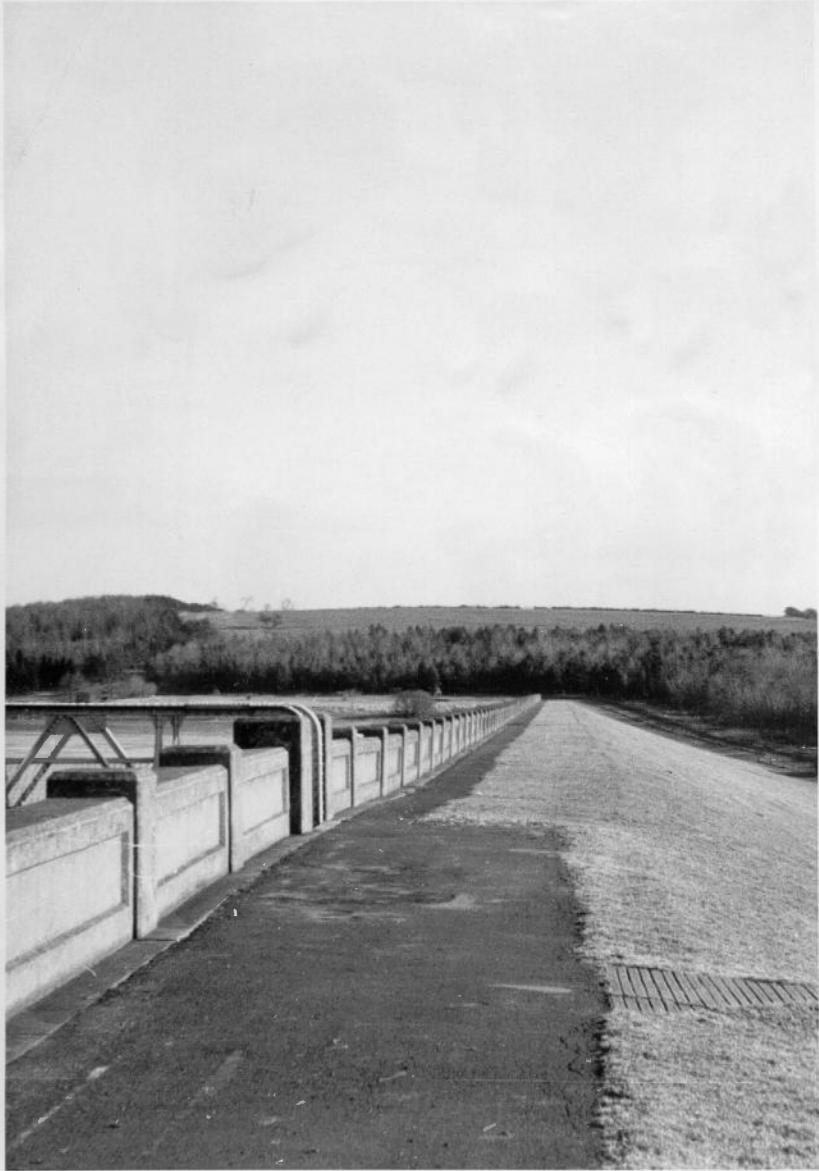
Eye Brook dam, showing subsidence, March 1963.
