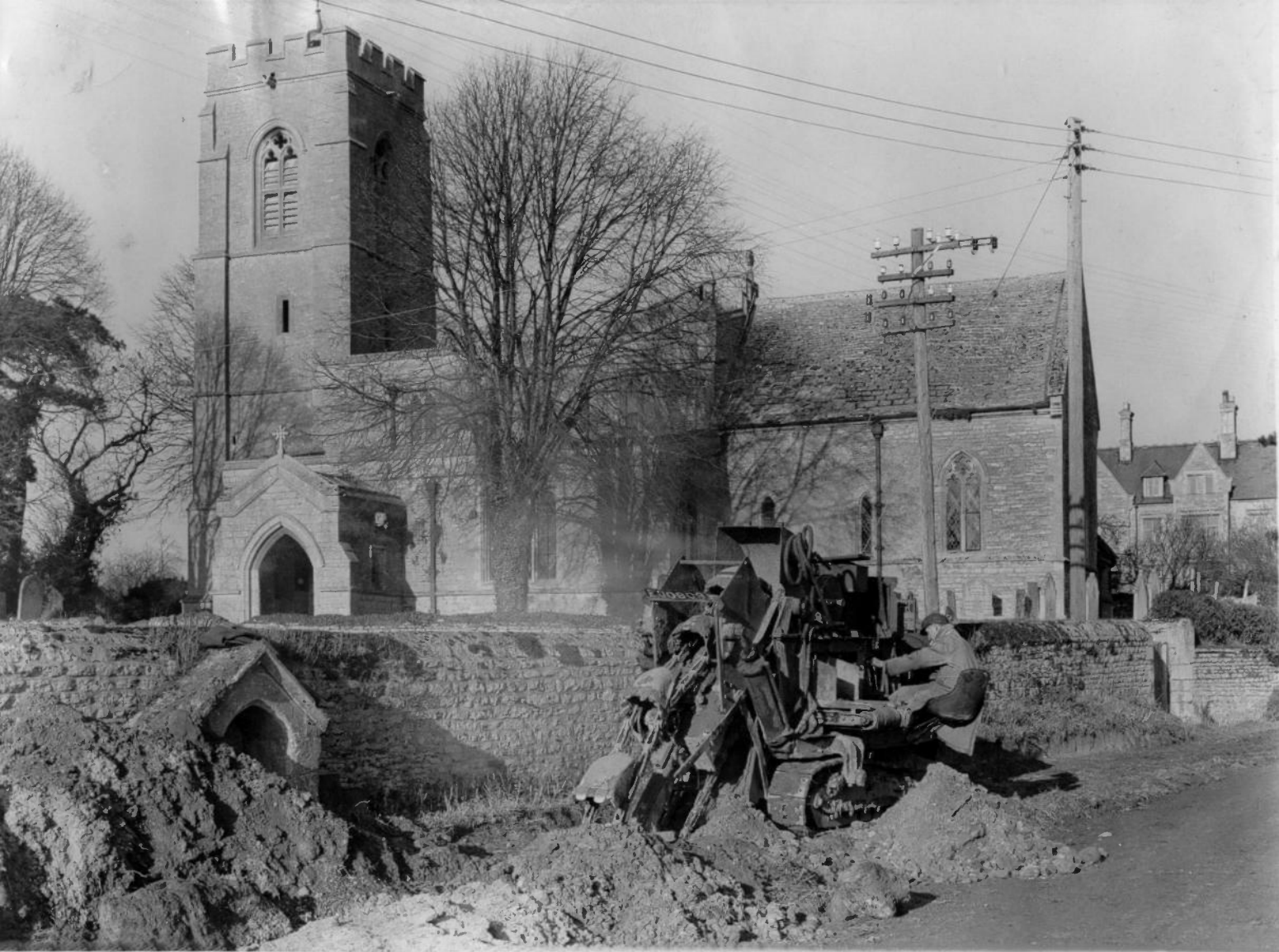
Crawshaw Robbins contractors, Allen Parsons digger at Little Oakley, digging 4" pipe trench. 1947.
